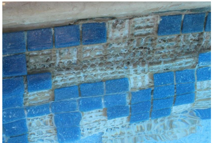
Figure 11. An example of mesh mosaic tiles that have failed at the waterline because of an inappropriate adhesive choice for a fibre-glass pool shell, but also because the mesh adhesive was water softening and obstructed the adhesive contact coverage with the tile itself.
